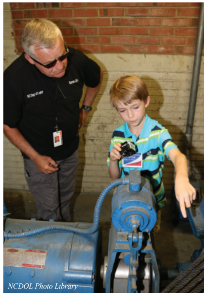
Cayden is shown the elevator mechanical room, above and below the elevator and Commissioner Berry's office at the Labor Building.
